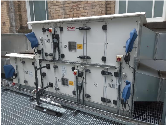
The CLIMACIAT Airaccess units cover all main areas of the hotel, offering exceptionally quiet operation.
