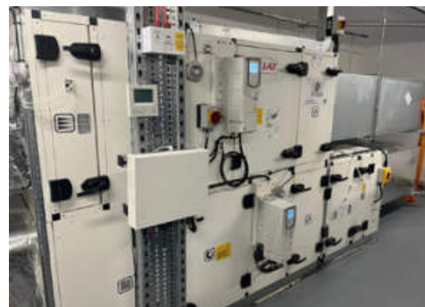
CIAT's AHU installed and integrated with Garsington Studios' Building Management System
