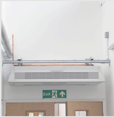
One of 7 above door-mounted CIAT MajorLine Fan Coil Units (FCUs).
